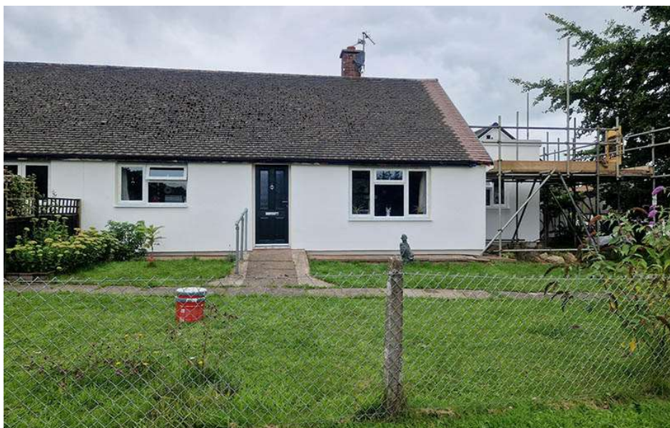
Figure 13 North Devon Homes property which received replacement cavity wall insulation, external wall insulation, flat roof insulation, new doors and high heat retention storage heaters under the Social Housing Decarbonisation Fund wave 1
